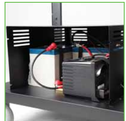
Integrated power system
