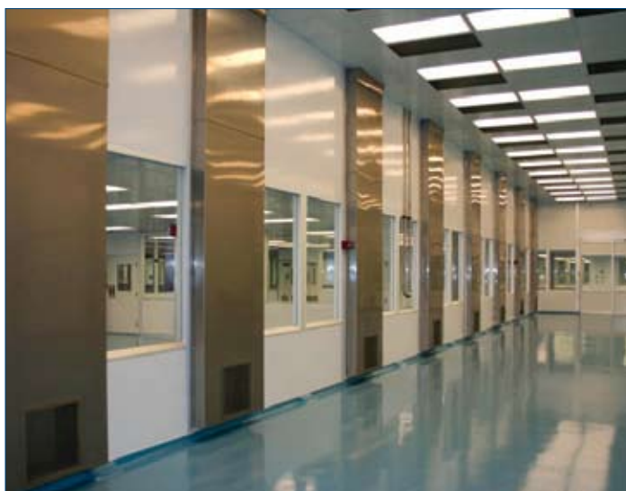
Duct work can be supported off walls for return air chases.
