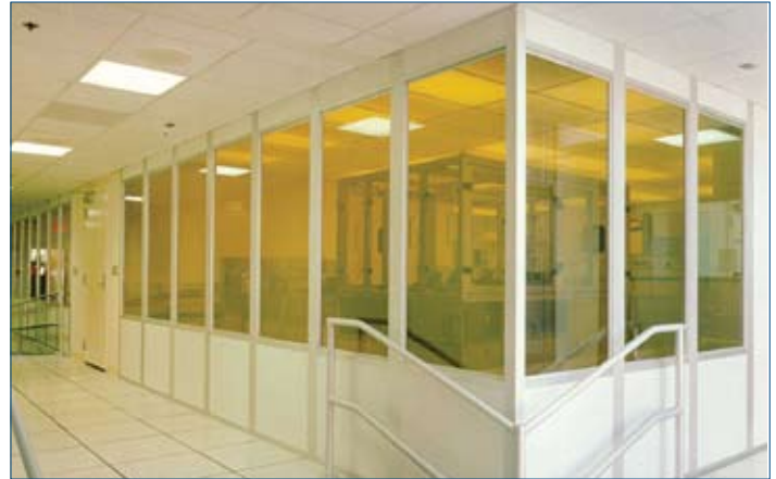
Special glazing has been flush glazed into walls to minimize ledges.
