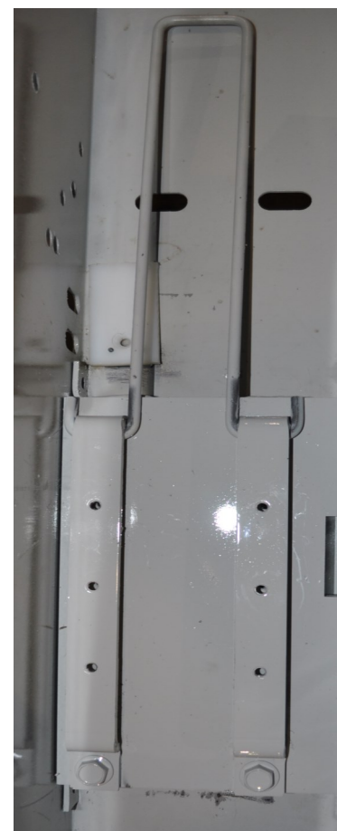
Fig 2. Safety brake deployed.
