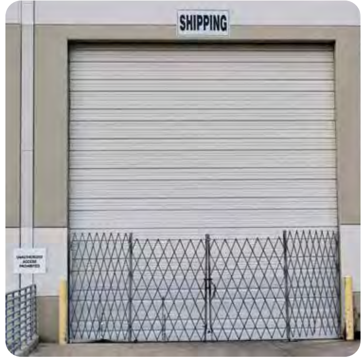
Above: folding gates let you keep overhead doors open, but still allow a measure of security.
