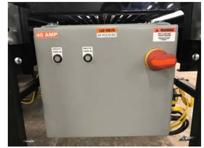
Figure 7: Power Panel with Disconnect Switch
