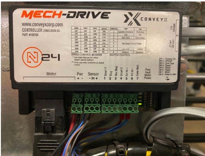
Figure 27: MECH-DRIVE ZoneLogix UL Drive Card wiring and lights during normal operation.
