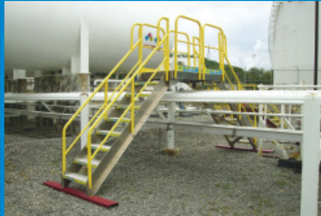
Eight stair pipe crossover.
