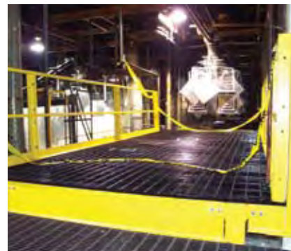
This conveyor access platform creates a secure area for maintaining this top hung conveyor system.
