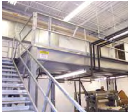
A galvanized candy processing equipment platform enables personnel to supply materials from above while maintaining floor space below for the candy making process.
