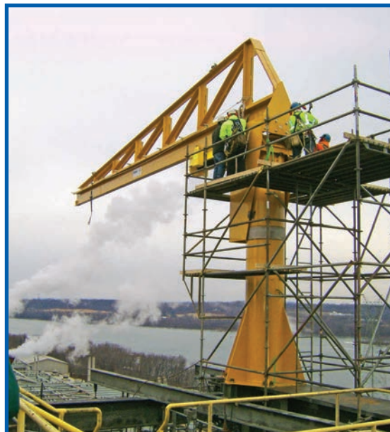
A 2-ton Spanco 100 Series Freestanding Jib Crane with a 50-foot span trussed boom. The crane is mounted to the existing structure of a coal plant on the Susquehanna River. It is used to replace large coils that are part of a steam duct system.
