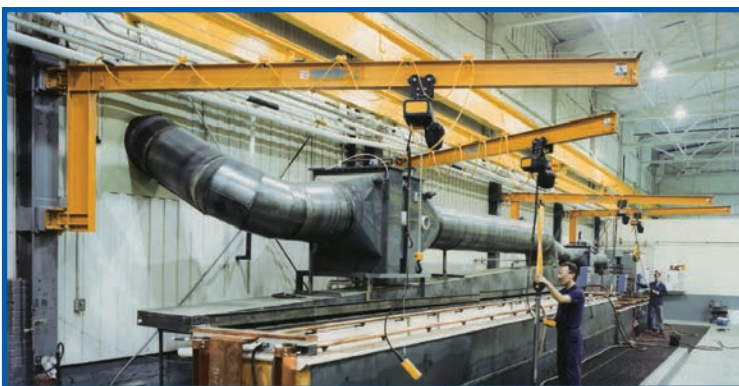
At this plant, four ¼-ton Spanco 300 Series Wall-Mounted Jib Cranes load and unload materials from a production bench. They can also transfer goods to adjacent cranes' coverage areas.
